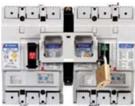
Slide Interlock Installed Between two MCCBs
